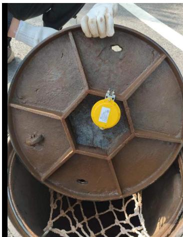
Iron manhole cover
