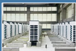
Multi-split Air Conditioner
